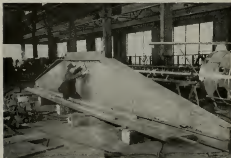
One of two strongbacks for the Ste. Helene under construction in Bethlehem's fabricating shops. These are to carry locomotives aboard the vessel.
